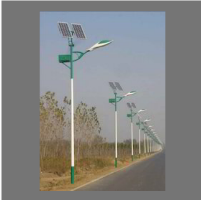
LED Solar Street Lighting System
