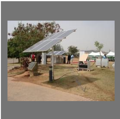
Solar Water Heating System
