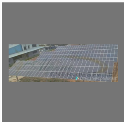
On Grid Solar Power Plant
