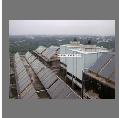
Industrial Solar Water Heating System
