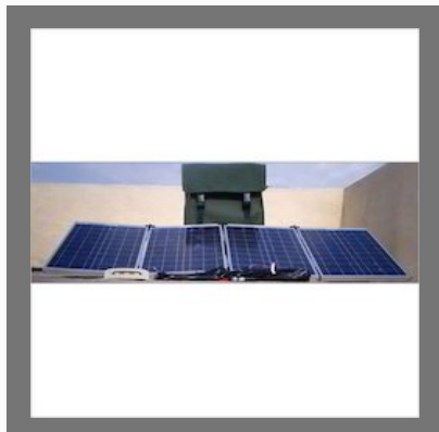
Solar Power Systems
