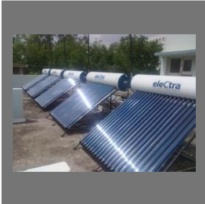
Electra Solar Water Heating System
